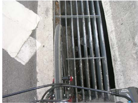
Bridges, with dangerous storm grates like this, can be hazardous.
